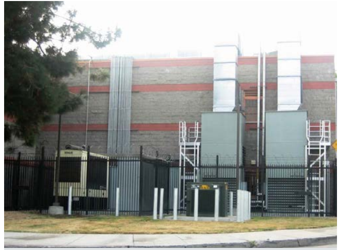
Figure 12. Ground-mounted fan with external ducting. Photo courtesy of Gladstein, Neandross & Associates, NREL 44703
