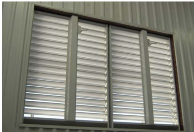
Figure 15. In-wall louver that provides make-up air flow. Photo courtesy of Gladstein, Neandross & Associates, NREL 44706
