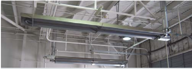
Figure 18. Gas-fired infrared tube-type heater needs to be replaced or removed. Photo from Gladstein, Neandross & Associates, NREL 44903
