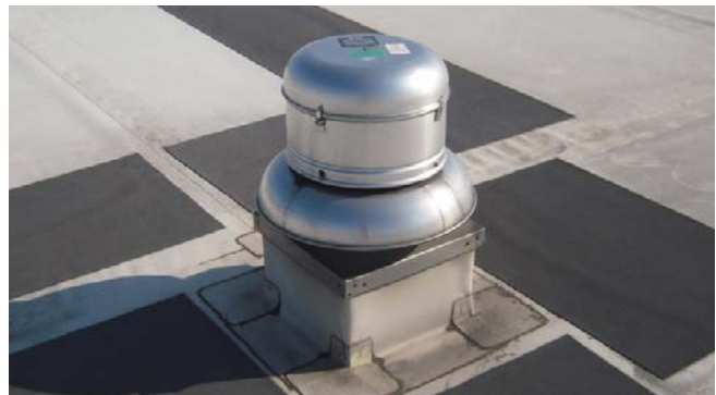
Figure 8. Roof-mounted upblast fan. Photo courtesy of Gladstein, Neandross & Associates, NREL 44698
