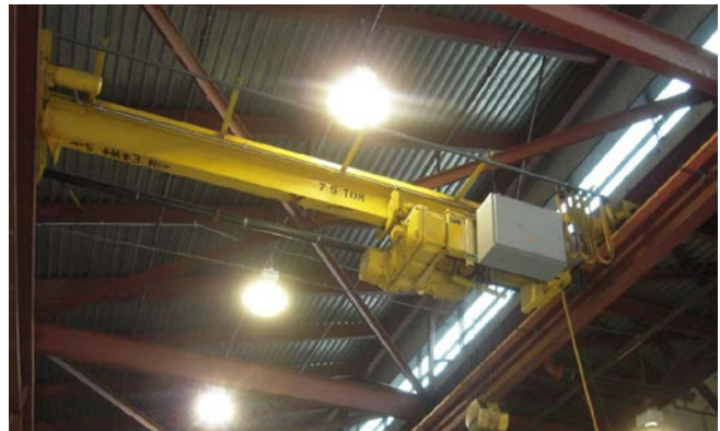
Figure 27. A typical overhead crane. Photo from Gladstein, Neandross & Associates, NREL 44681
