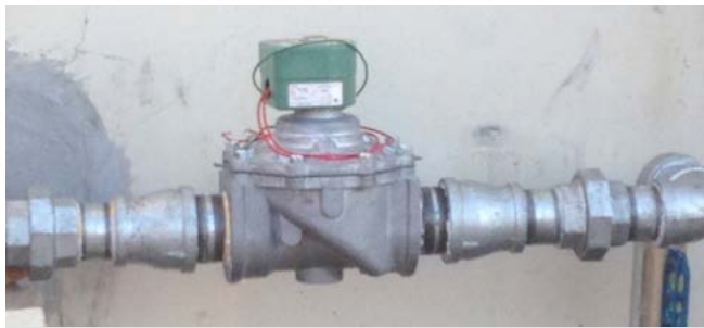
Figure 41. Electrically controlled main gas shut-off valve. Photo from Gladstein, Neandross & Associates, NREL 44892
