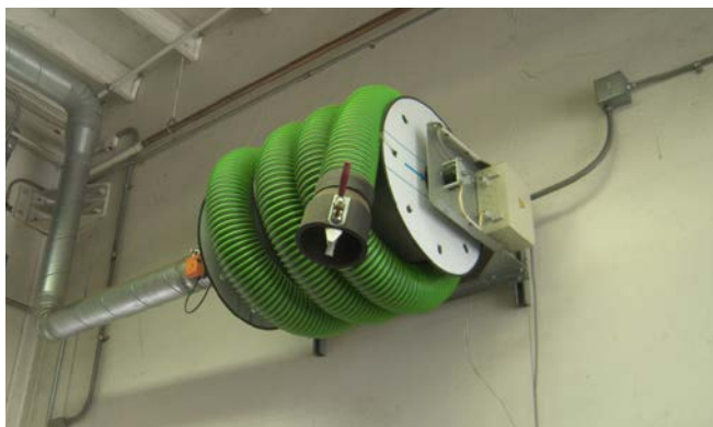
Figure 38. The exhaust from a natural gas engine is hotter than that from a diesel engine, so some exhaust extractor hoses may need to be replaced during the facility modifications. Photo from Gladstein, Neandross & Associates, NREL 44695
