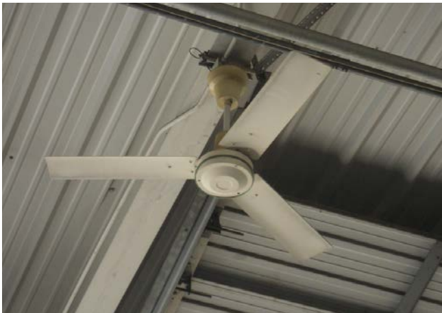
Figure 25. An overhead rotary fan that presents a potential ignition source. Photo from Gladstein, Neandross & Associates, NREL 44679
