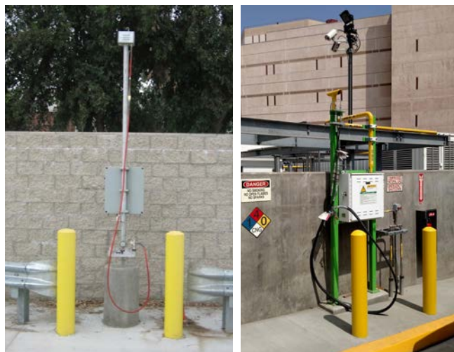
Figure 36 (left). A defueling post.
