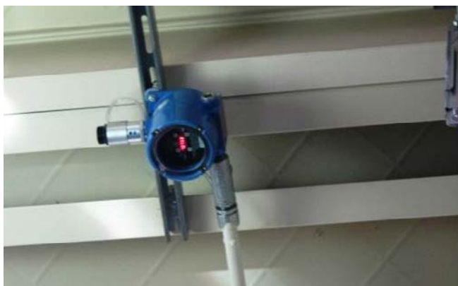
Figure 29. A ceiling-mounted combustible gas detection head. Photo from Gladstein, Neandross & Associates, NREL 44683
